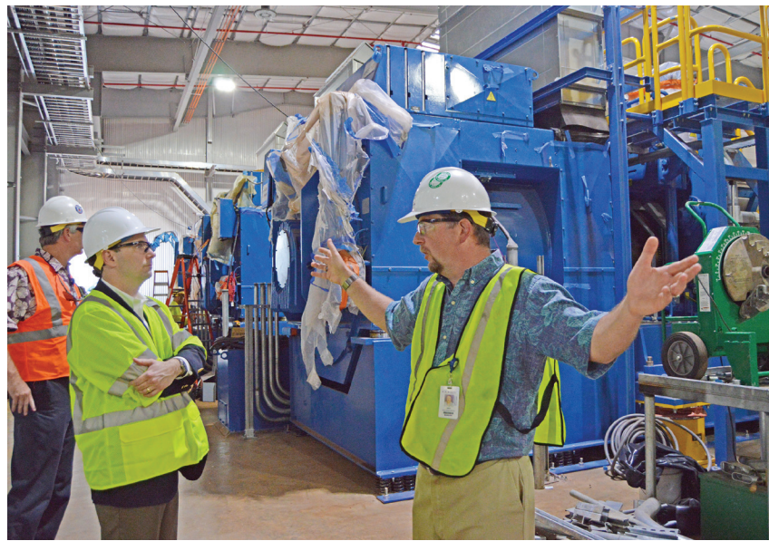
Acting Assistant Secretary of the Army for Installations, Energy and the Environment Jordan Gillis listens to Hawaiian Electric Co. Manager of Generation Project Development Jack Shriver on 19 January 2018 during a tour of the Schofield Barracks Generating Station (U.S. Army photo by Karen A. Iwamoto, Oahu Publications).
