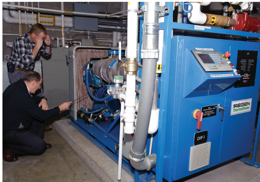
A.J. Ballard, the energy manager for the Maine Army National Guard, points out some of the engine details of the award-winning combined heat and power system at the Maine Army National Guard Army Aviation Support Facility in Bangor, Maine. "This is a wonderful machine," said Ballard. "This system produces electricity we don't have to pay for, and heat we don't have to pay for" (U.S. Army photo by Staff Sergeant Angela Parady, 121st Public Affairs Detachment).
