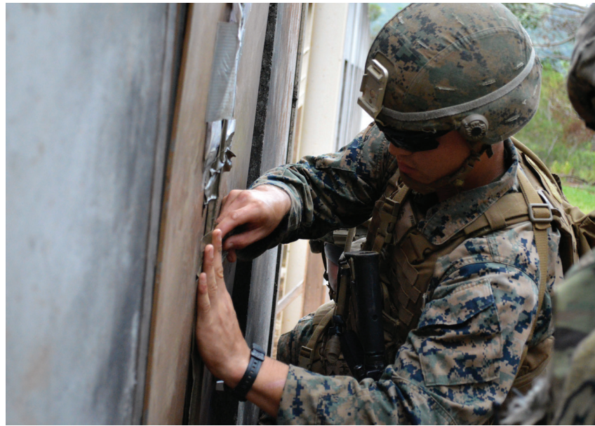
A Marine from the 2nd Battalion, 3rd Marine Regiment, based out of Marine Corps Base Hawaii Kaneohe Bay, places a demolition charge on a door at Schofield Barracks, Hawaii, on 30 August 2017. Army combat engineers and Marines trained together on a variety of door breaching techniques. (U.S. Army photo by Staff Sergeant Armando R. Limon, 3rd Brigade Combat Team, 25th Infantry Division)
