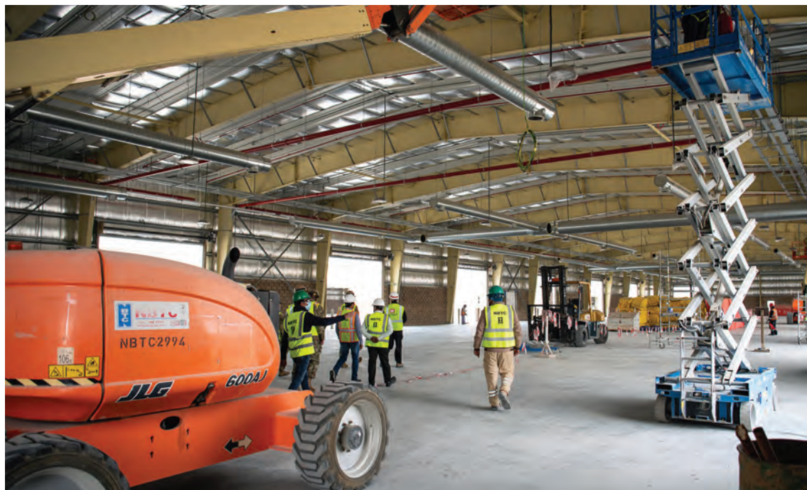
A team from the U.S. Army Corps of Engineers walks through one of five Army prepositioned stock buildings currently under construction at Camp Arifjan, Kuwait, on 31 January 2022. When completed, the five facilities will provide critical environmental protection for Army Materiel Command's pre-positioned stock, part of a U.S. Army program in which equipment sets are stored around the globe for use when a combatant commander requires additional capabilities (U.S. Army photo by Richard Bumgardner).
