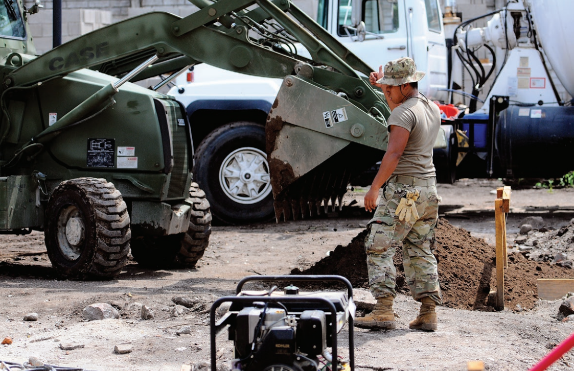
Pvt Sair Silverio, an engineer with the 926th Engineer Brigade, 844th Engineer Battalion, 390th Engineer Company out of Chattanooga, Tennessee, serves as a ground guide to one of his colleagues operating a High-Mobility Engineer Excavator at the Canton El Amate engineer site during the humanitarian assistance exercise Beyond the Horizon (BTH) in Zacatecoluca, El Salvador. BTH is a Southern Command, U.S. Army South led exercise in which personnel construct schools and clinics and provide medical, dental and veterinary support. (National Guard photo by Staff Sergeant Angel D. Martinez-Navedo)
