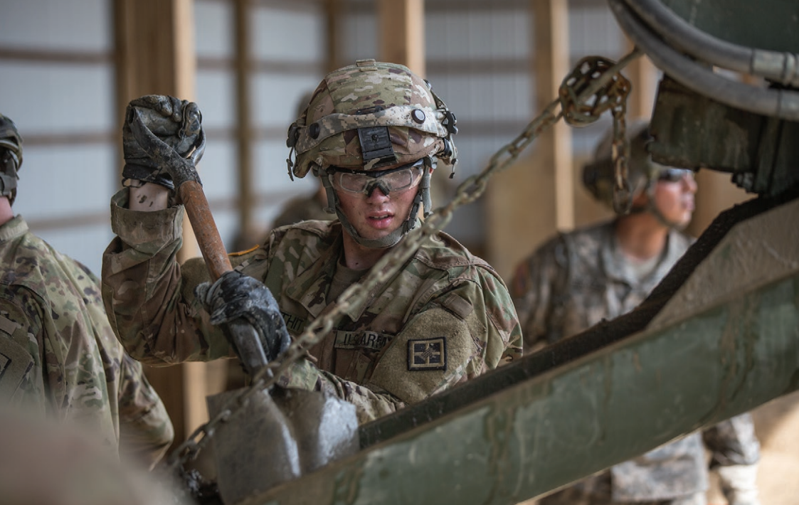
U.S. Army Reserve Private First Class Devon Douthit, 465th Engineer Company, 416th Engineer Command, shovels concrete from the chute of an M5-Concrete Mobile Mixer during Combat Support Training Exercise (CSTX) 86-18-02 at Fort McCoy, Wisconsin, 16 August 2018. The CSTX exercise is a large-scale training event where units experienced tactical training scenarios specifically designed to replicate real-world missions (U.S. Army Reserve Photo by Specialist John Russell).
